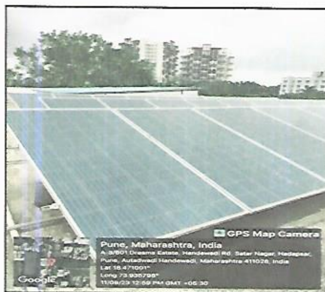
Photograph of Roof Top Solar PV Plant:
